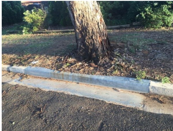
Photograph 10: Retention of Eucalyptus robusta at Bellbird Way through the installation of a formed steel gutter over the structural root zone.
