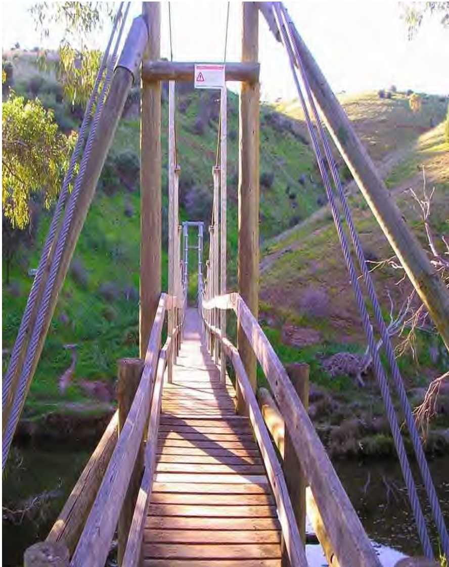
The Old Noarlunga Swing Bridge (before replacement) which was successfully replaced by 'Moodie' after a successful Community campaign to retain a similar 'suspension' style bridge rather than replace it than a 'fixed' modern bridge (This bridge is very similar to current the Wellington suspension bridge)
