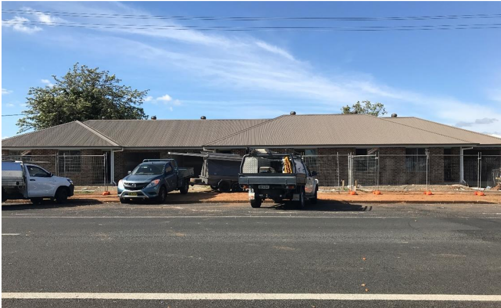
Figure 4: Northern building elevation of the previously approved units currently under construction (image taken 1 December 2017).
