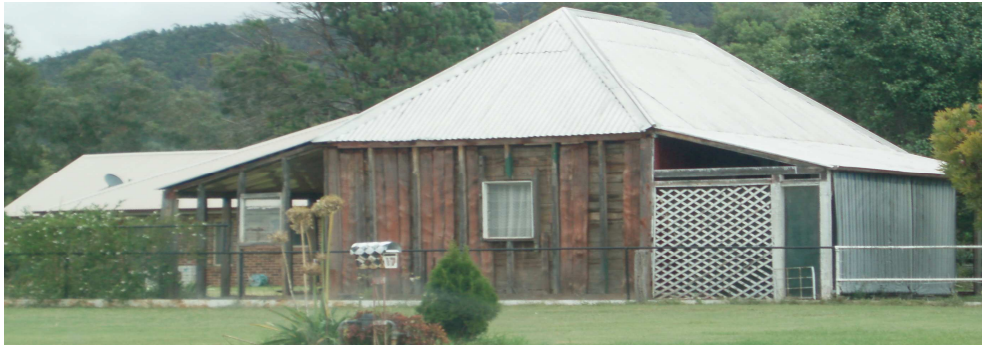
Figure 20: Slab construction with original timber shingles underneath iron roof (circa 1860's), 21 Sutton Street (Source: Strong, 2011)
