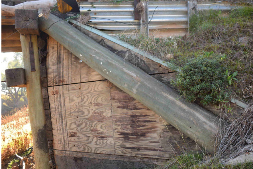
Figure 3-16 Abutment pile rotation (Source: FBE)
