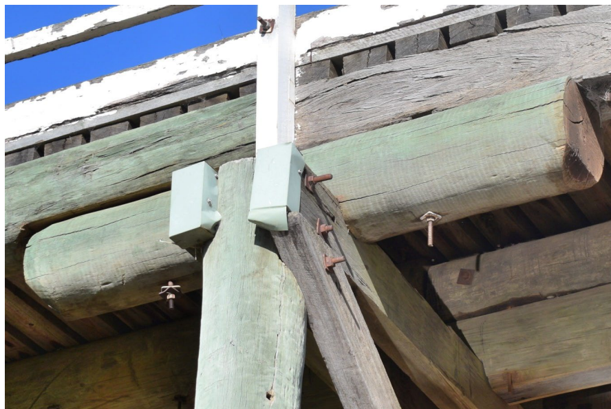
Figure 3-11 Corbel - loose bolted connection with main girder (Source: FBE)
