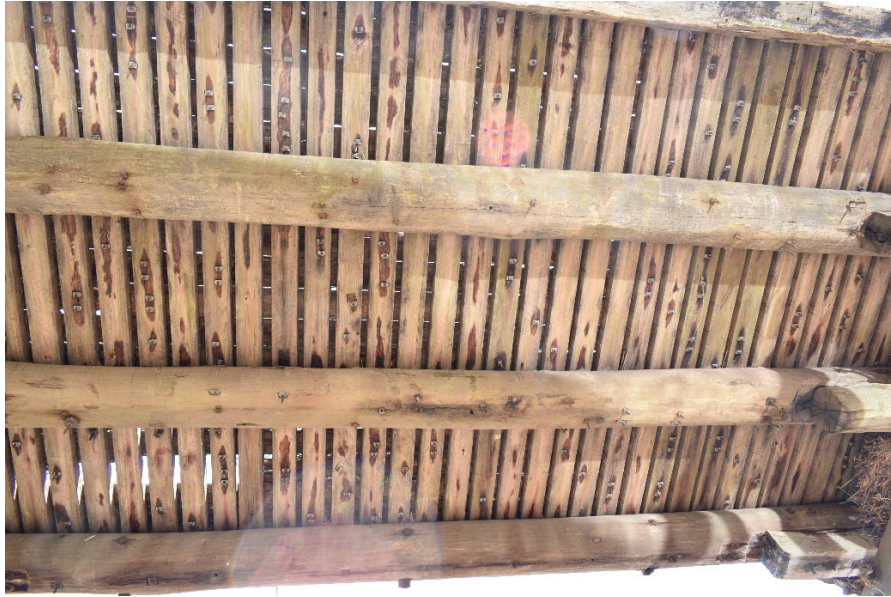
Figure 3-5 Transverse planks, typical condition (Source: FBE)
