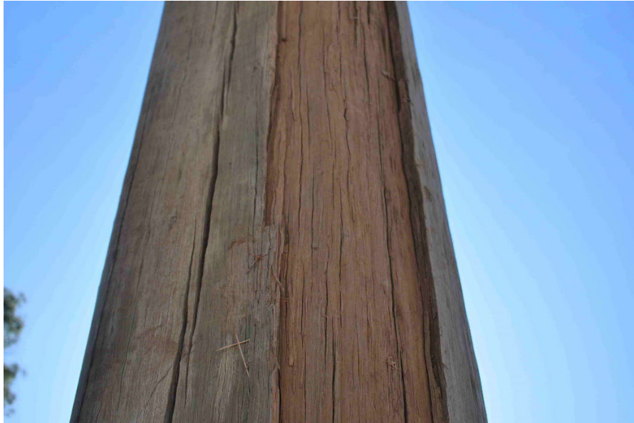
Figure 3-13 New pile with evidence of outer layer delamination (Source: FBE)
