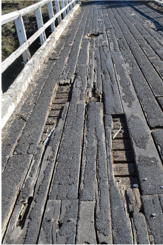
Figure 3-7 Typical top of deck condition (Source: FBE)
