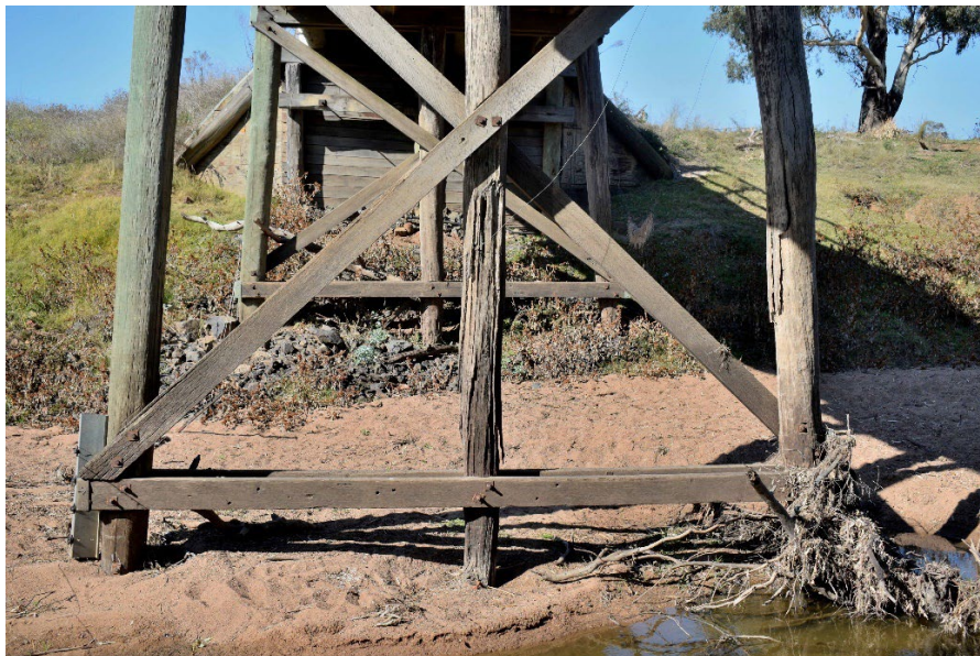
Figure 3-14 Typical deterioration of piles with section loss (Source: FBE)
