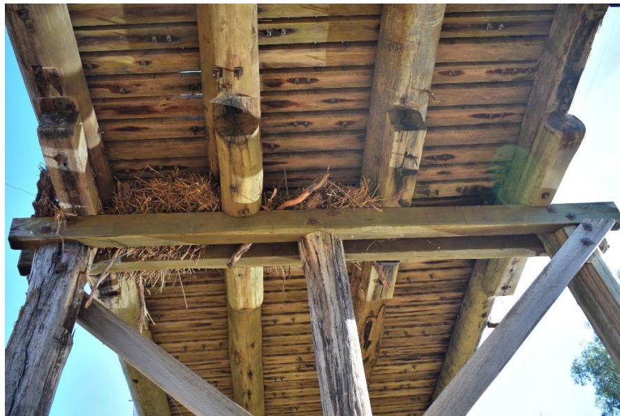
Figure 3-10 Corbels - typical condition - note flood debris (Source: FBE)
