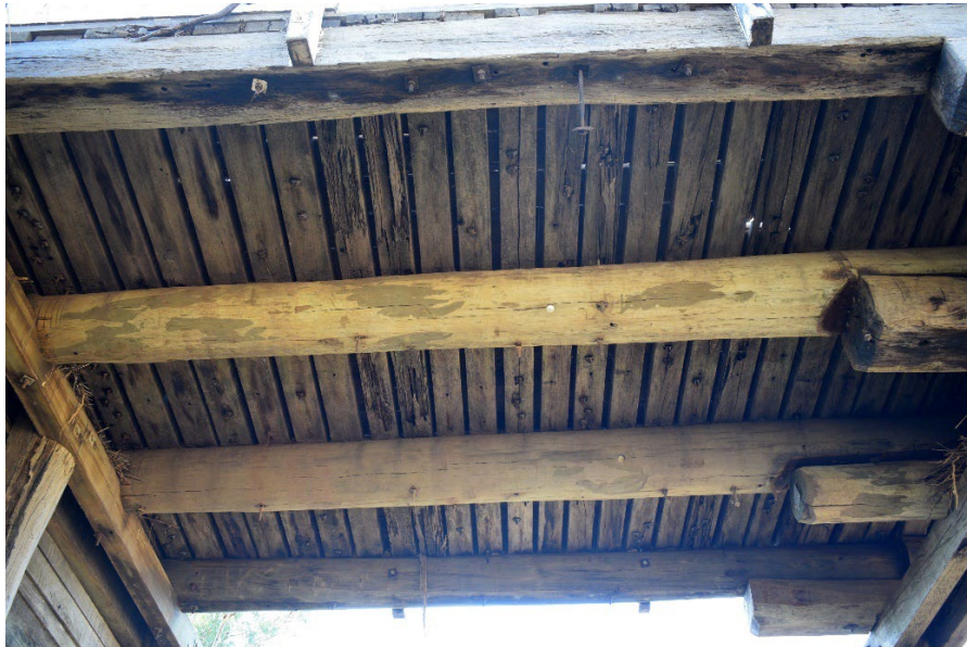
Figure 3-6 Transverse planks in poor condition at Span 1 (Source: FBE)
