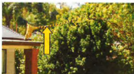
Insulated matting and tiger tail fitted to overhead service line
