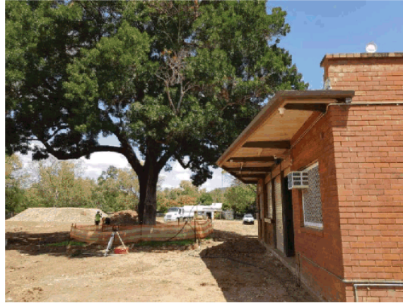
Plate 3. Looking from the east side of the building to the west. Photo shows the amount of excavation encroaching into the TPZ.
