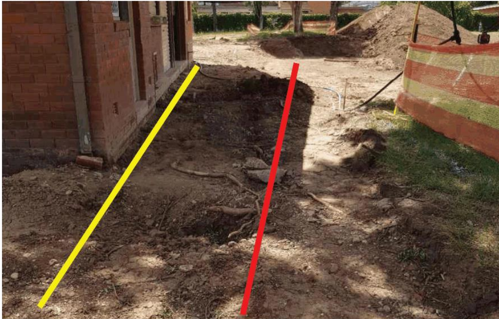
Plate 4. Roots damaged and encroachment in to TPZ and SRZ
