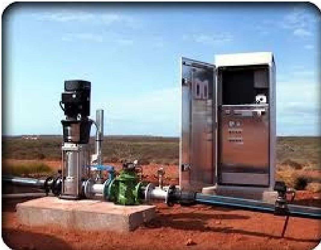
Figure 5-1: Typical bore water pump station
