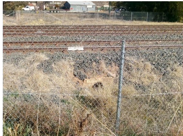
Photo 4-8: Culvert under the railway near the intersection of Narragal St and Douglas St
