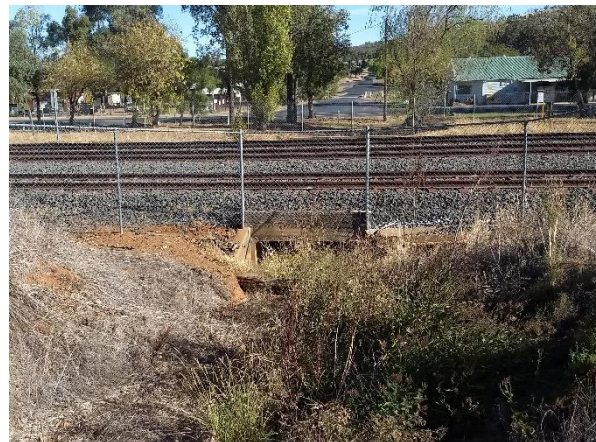
Photo 4-10: Culvert under the railway near the intersection of Narragal St and Chambers St
