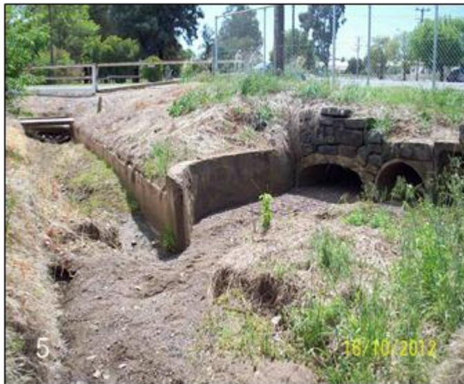
Silted channel downstream of intersection of Maxwell Street and Railway Avenue
