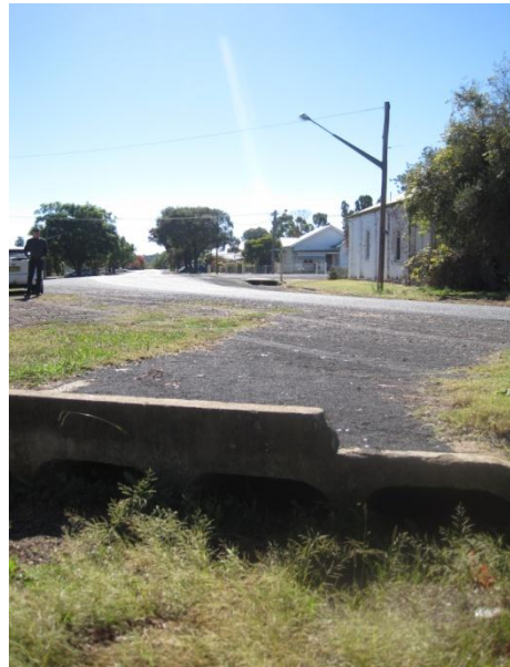
Silted culverts at outlet near intersection of Swift and Kennard Streets
