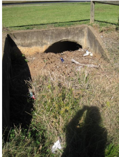
The silted culvert headwall inlet north (upstream) of Maxwell Street in Apex Park
